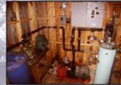
4. ...to a small collecting tank in a pumphouse...
